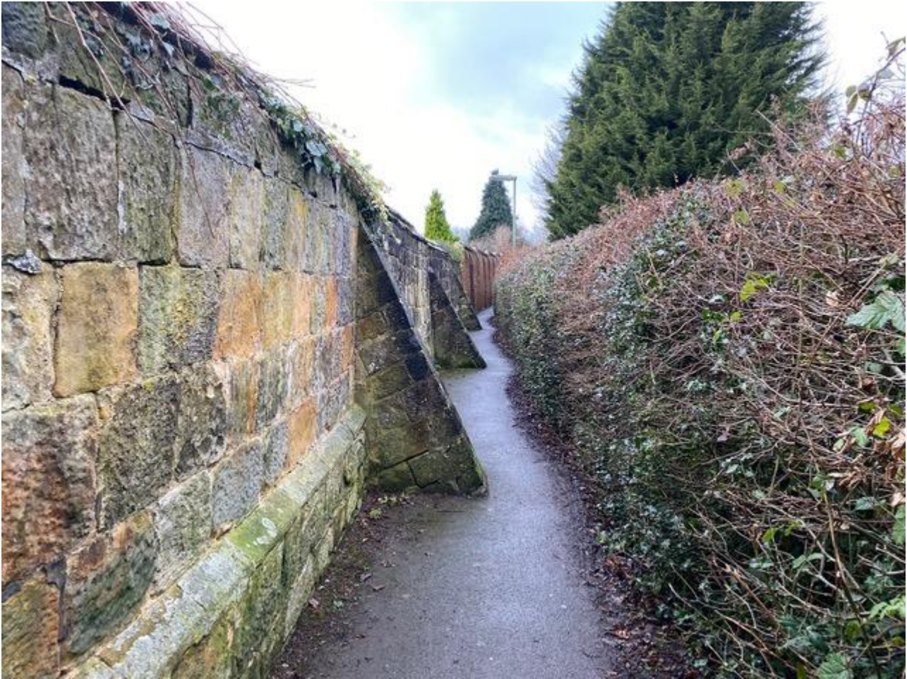
Figure 5 – The footpath, looking west, with the listed garden wall of New Place to the left.
