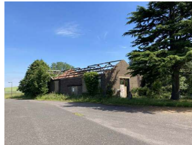
View of derelict former workshops
