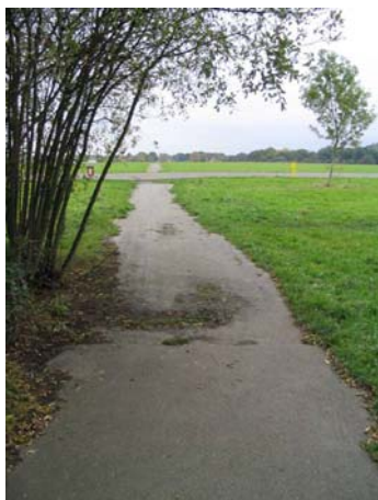
Left: The original Hayes Lane still crosses the airfield. Right: Existing Guard House. Below: View of the perimeter track, airfield and treed boundary.
